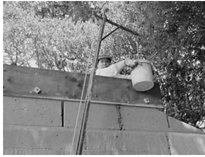
Jin Ling setting up and filling the Smartform system for the walling.
