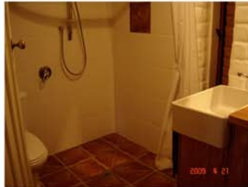
wet room (sloping tiles over water proof membrane to the floor waste, toilet pan behind door = good space for wheelchair access)
